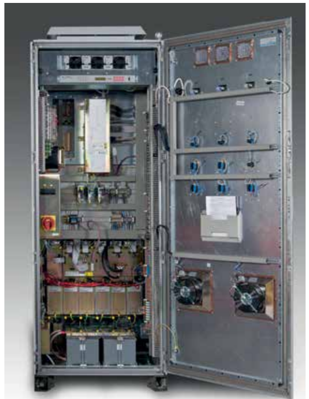
Figure 2: Inside a digital control cabinet for an active magnetic bearing system
