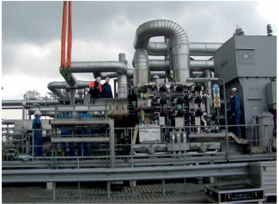
Figure 5: NAM motor (right) and compressor bundle (left) being installed at the Groningen site
